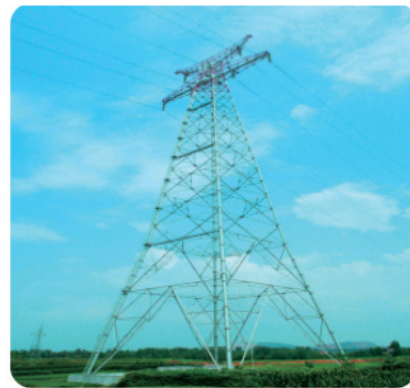
电力塔架 Electric transmission tower
