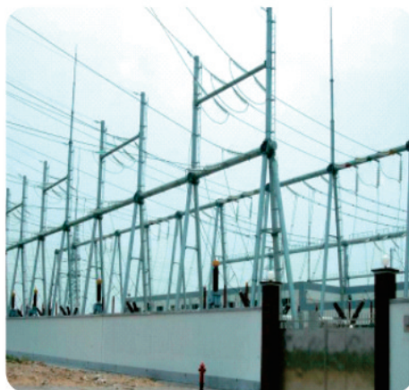
变电站构架 Trasformer substasion structure
