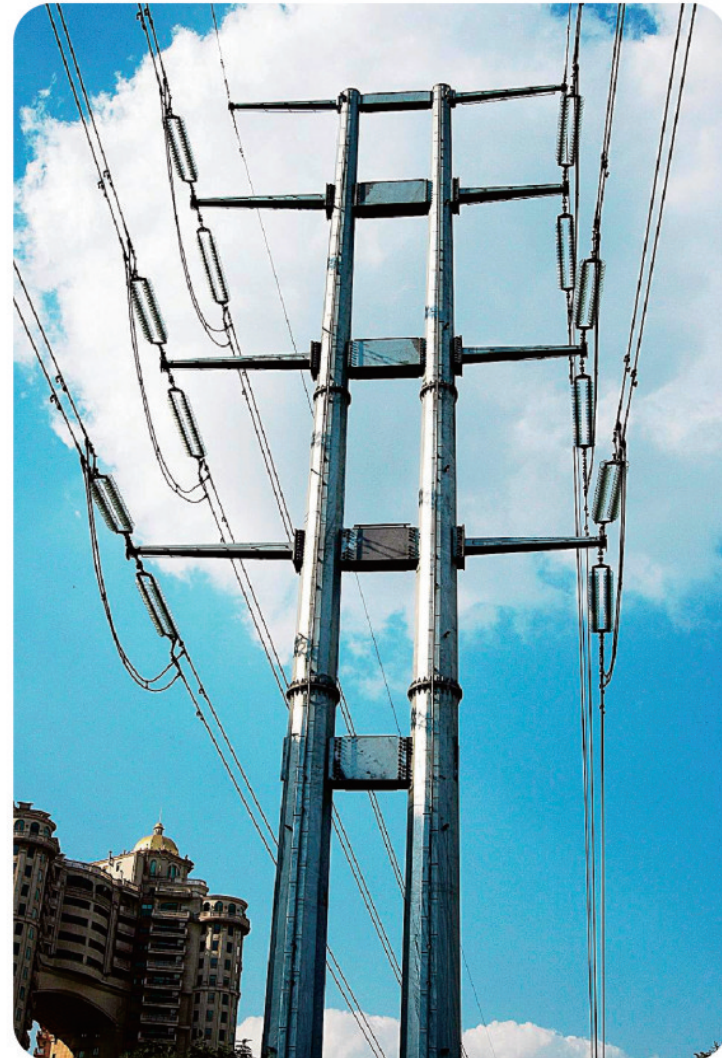
输电杆塔 Transmission pole
