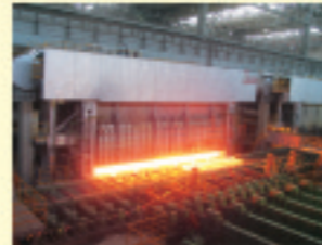
步进式加热炉 Walking beam reheating furnace
