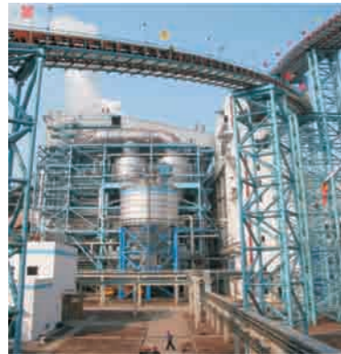
电站锅炉 Power plant boiler
