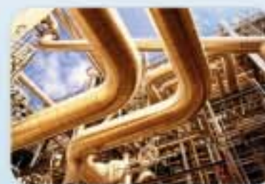
传送管道 Petroleum delivery pipeline
