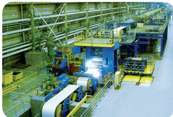
冷轧卷退火酸洗线APL(C) Cold-rolling Coils Annealing and Pickling Line
