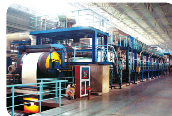
热轧卷退火酸洗线APL(H) Hot-rolling Coils Annealing and Pickling Line
