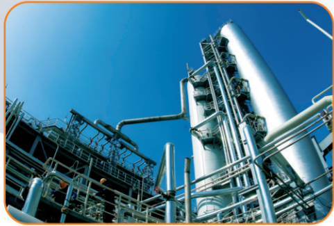
煤化工 Coal Chemical industry
